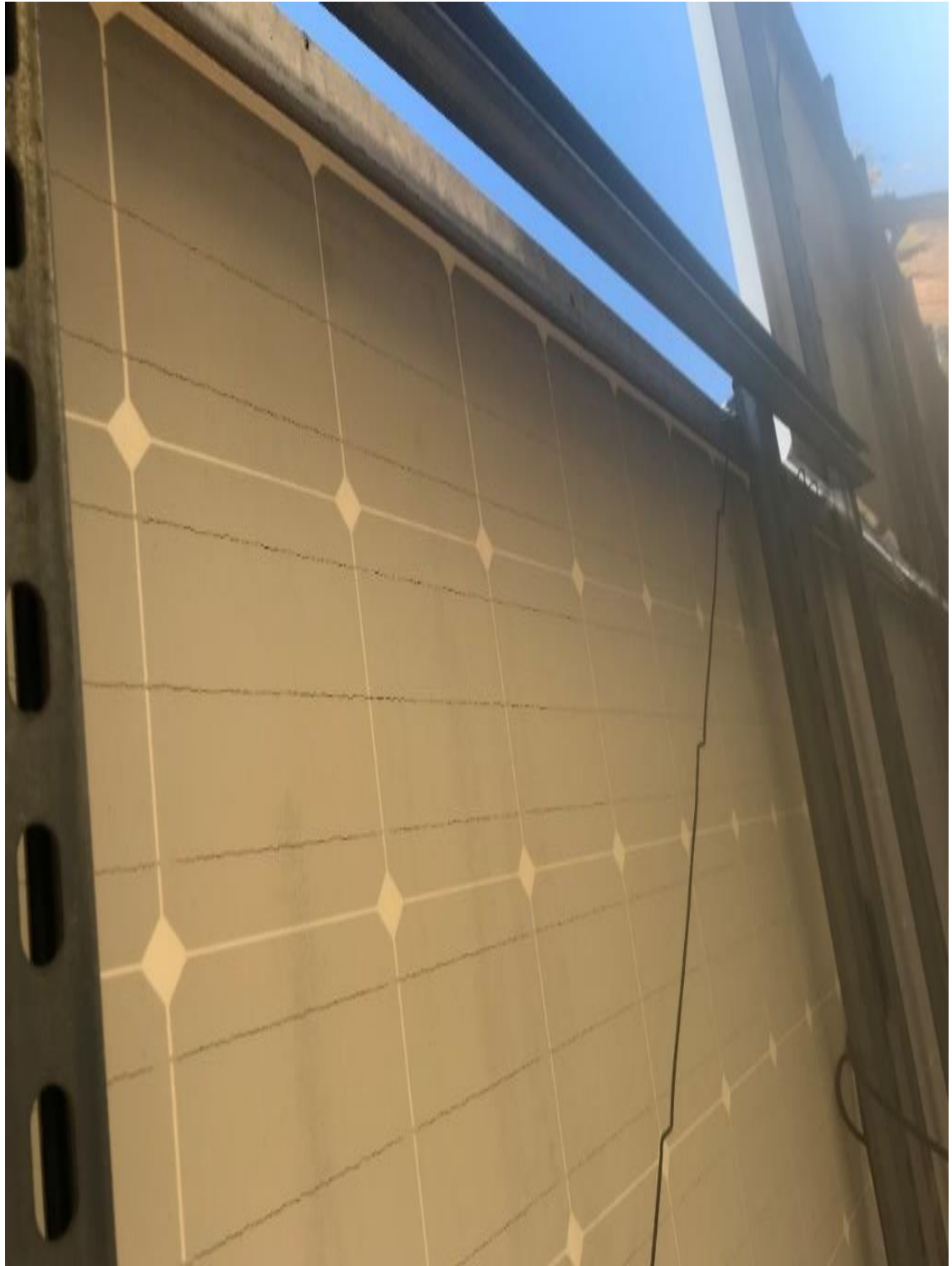
Cracked Backsheet Running the Length of the Bosch Solar c-Si M 60 NA30119 Module at the Rojas Property
